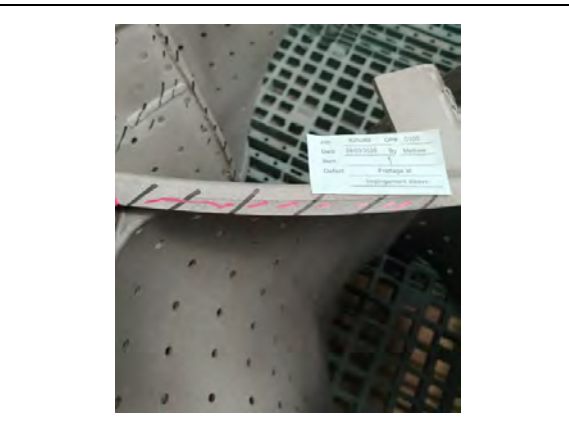
Fig.28 Fretting on impingement sleeve.
